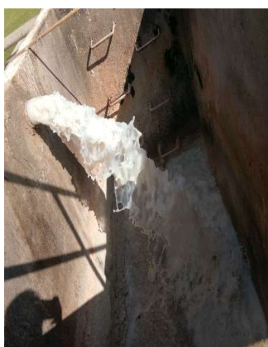
(a): Sampling Point (Inlet, ETP, Jaipur Dairy)
