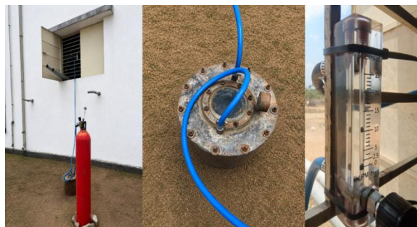
Fig.-3: Hydrogen Supply, Safety and Flow Metering Arrangement
