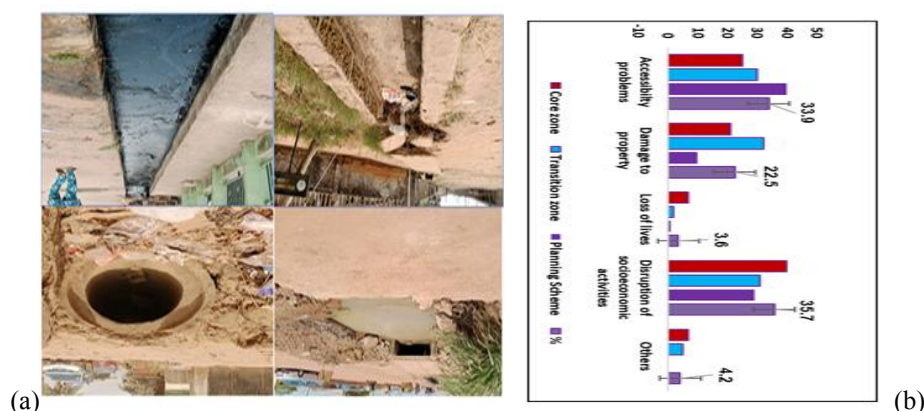
Fig.-3: (a) Existing Drainage Condition (b) Impact of Drainage Deficiencies in the Environment
